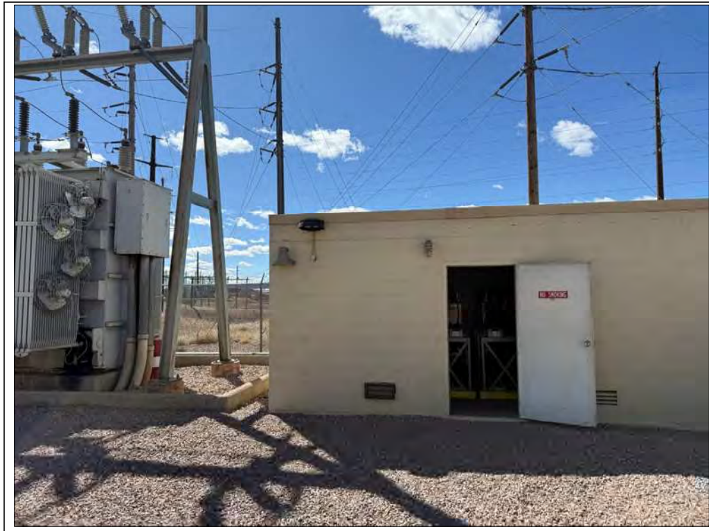
Photo 11: Building located west of the natural gas-fired generators housing a battery bank.
