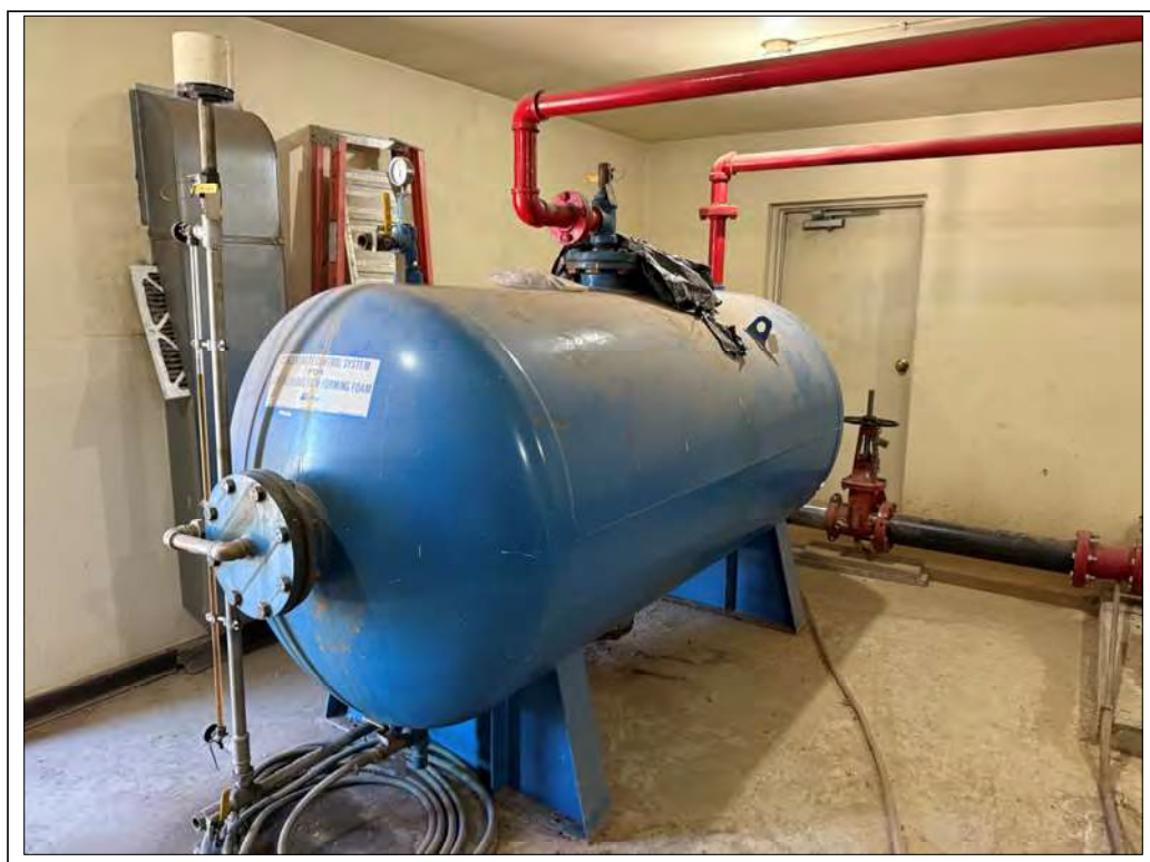
Photo 14: AFFF AST located in small building east of the 1,000,000-gallon ASTs.
