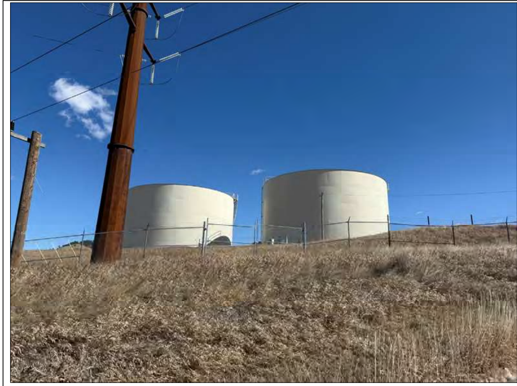
Photo 1: 1,000,000-gallon diesel ASTs near south boundary of Subject Property looking east.
