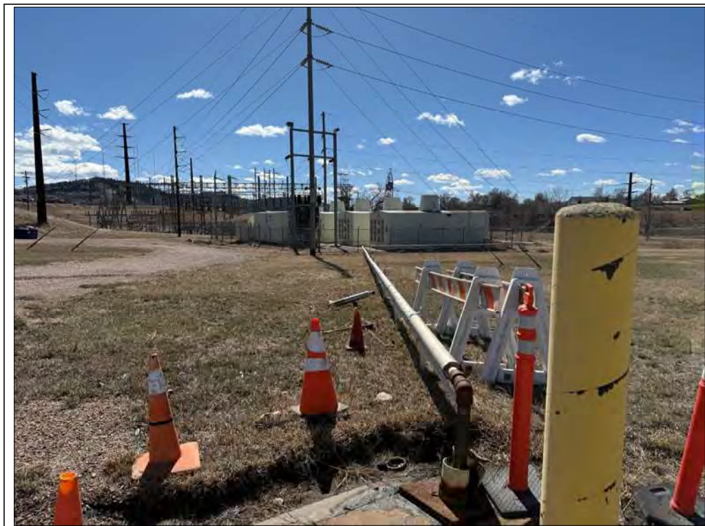
Photo 16: Example of above ground piping connecting the 31,000-gallon diesel AST to the diesel generators.
