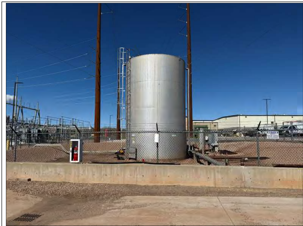
Photo 4: 31,000-gallon diesel AST and containment looking north.
