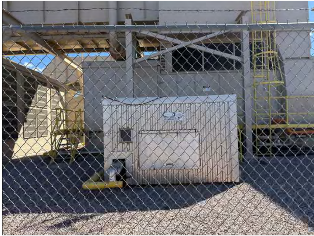
Photo 9: Backup diesel fuel AST attached on the north side of each of the natural gas-fired generators.
