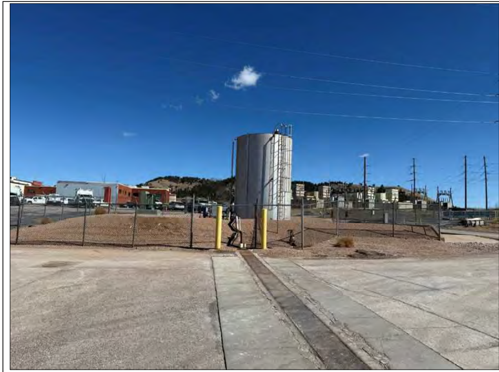
Photo 5: 31,000-gallon AST and fuel distribution piping/trench looking east.
