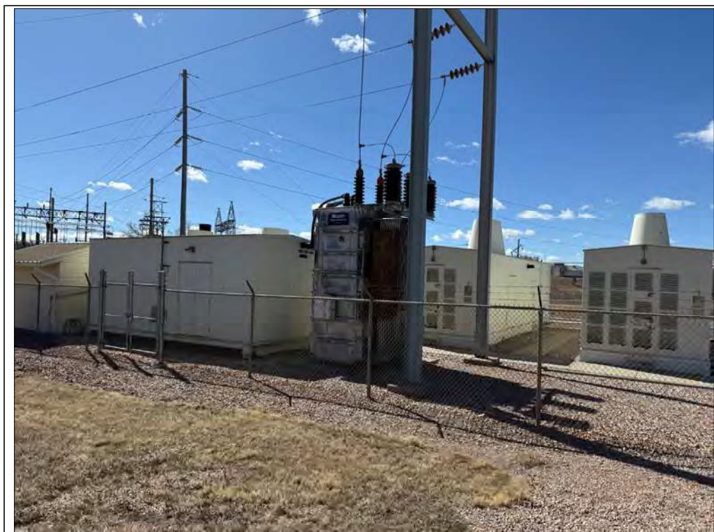
Photo 6: Five diesel-fired generators and associated sheds/equipment near the west boundary of the Subject Property looking southwest.
