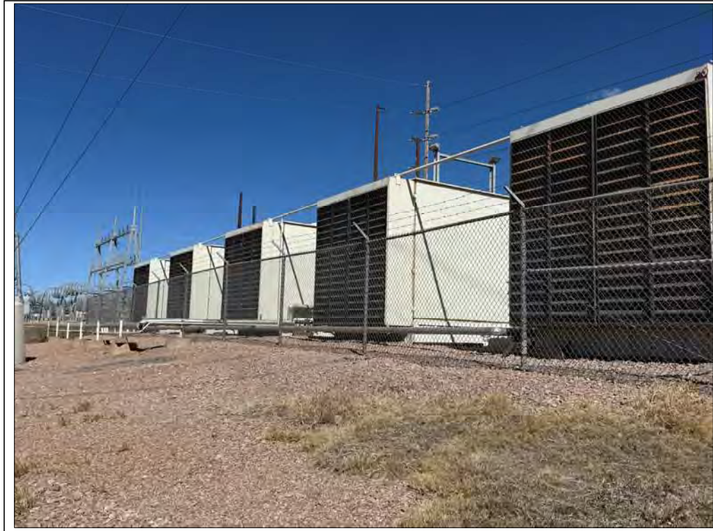
Photo 7: Five diesel-fired generators looking north.
