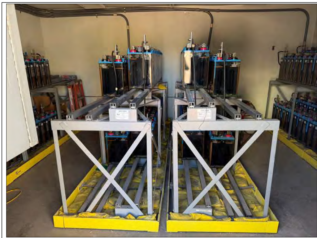
Photo 12: Batteries with spill containment located in small building near the natural gas fired generators.
