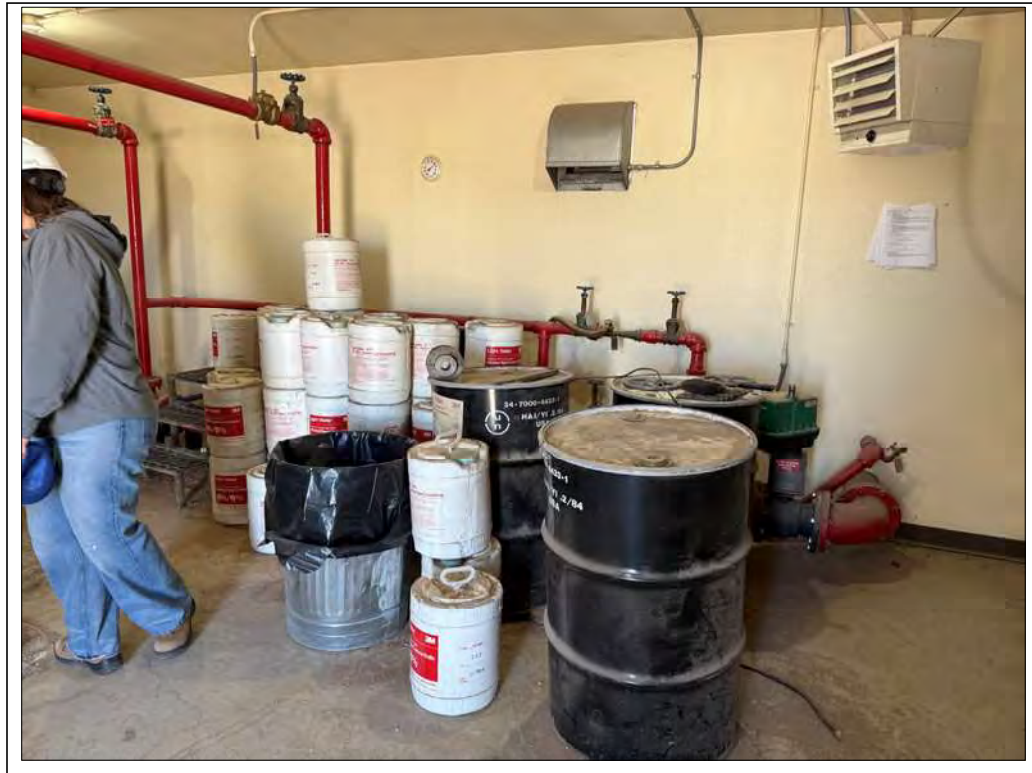
Photo 13: AFFF containers in small building east of the 1,000,000-gallon ASTs.
