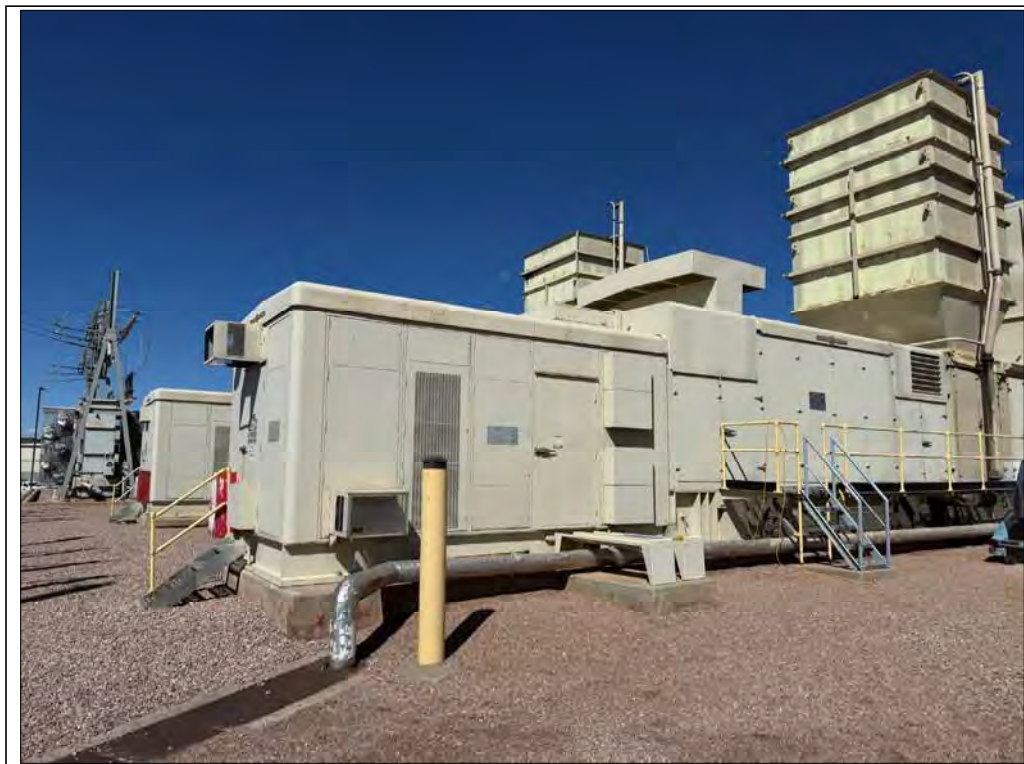
Photo 8: West end of natural gas-fired generators looking north.
