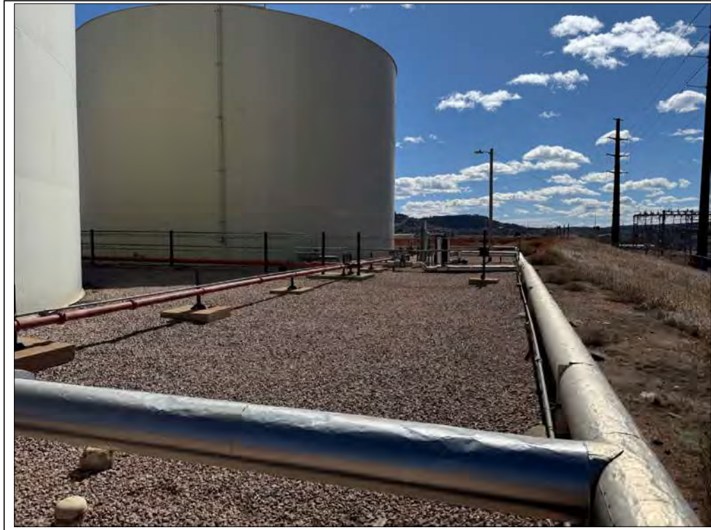
Photo 15: Example of above ground piping connecting the 1,000,000-gallon diesel ASTs to the natural gas generators.
