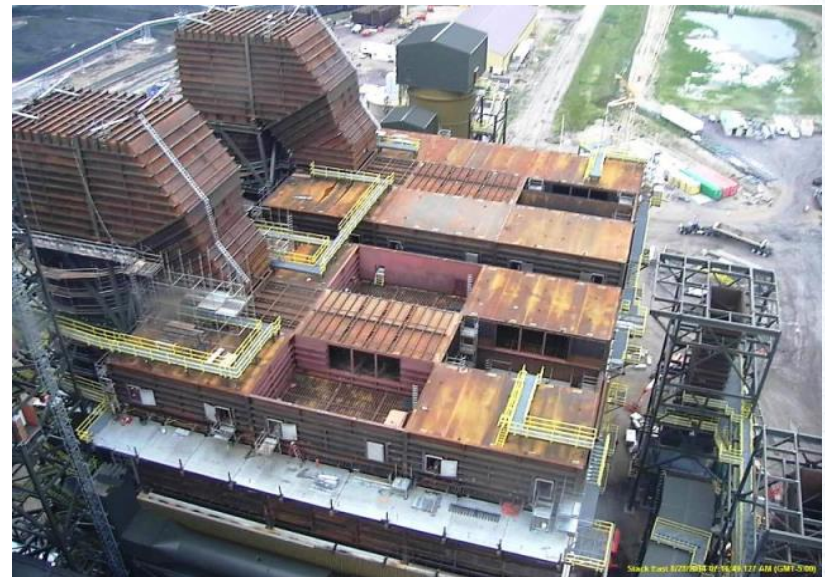
2014-08-29 CFB & baghouse top view
