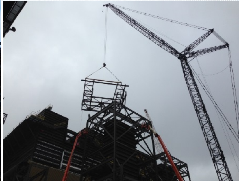
2014-08-29 ID fan duct support steel – Notice IW on top beam!
