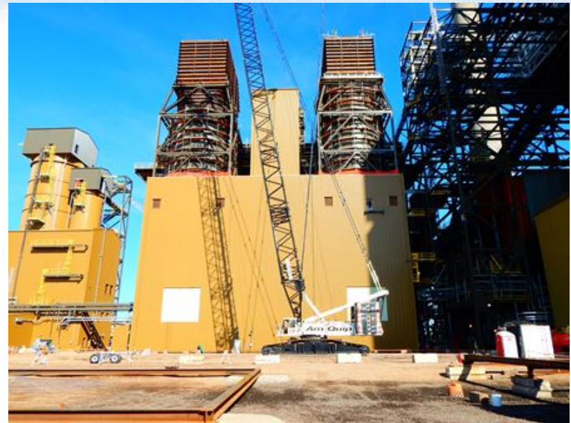
2014-08-27 Plant southwest view, WA/PL, CFB, S SCR
